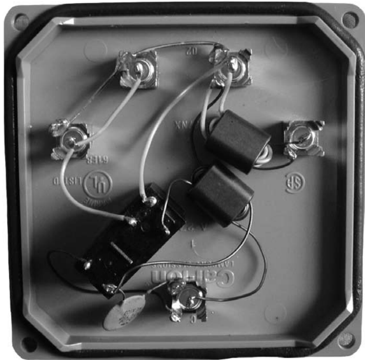
Figure 12 — End-fire directional control built into the cover of a “marine grade” plastic electrical box. Be sure to drill holes in the box to allow moisture out.
